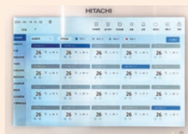
New air conditioner control panel
